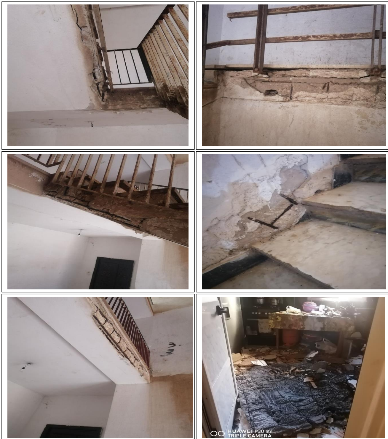
Figure 2. Dilapidated buildings of the neighborhoods under study from inside and outside (Source: [13])
